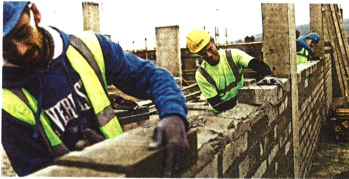
Construction workers in Dublin. Housebuilding in Ireland has increased and commercial property transactions have doubled in the past year – Chris Ratcliffe/Bloomberg
